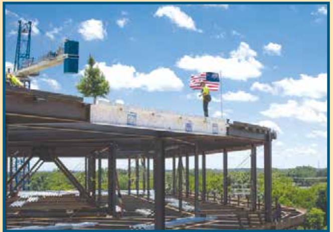
The final steel “beam of hope” was set in place during a topping out ceremony in June.
