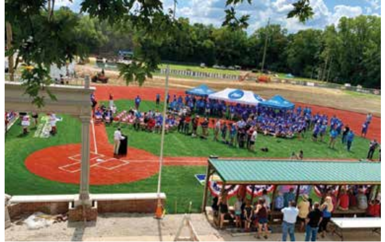
More than 200 St. Elizabeth associates volunteered to renovate the new Bellevue Vets ball field complex in conjunction with the Reds Community Fund.
